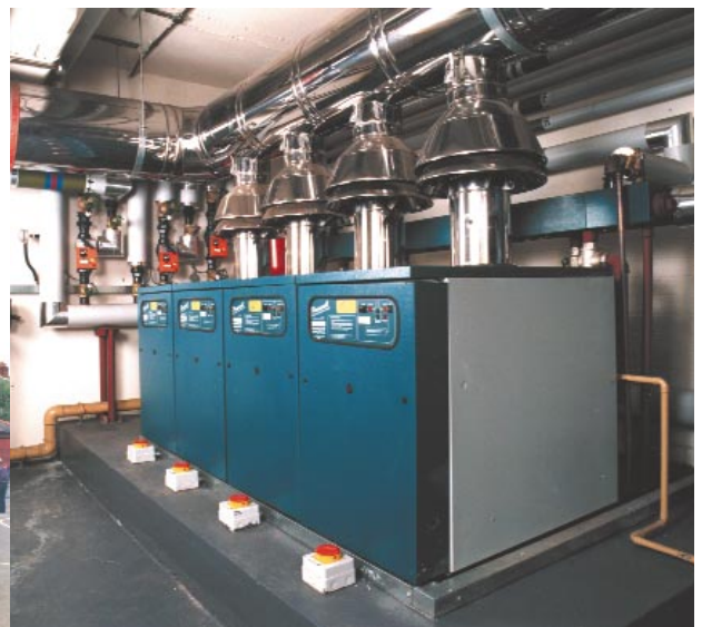
Figure 2 The new modular boiler at Church Road
