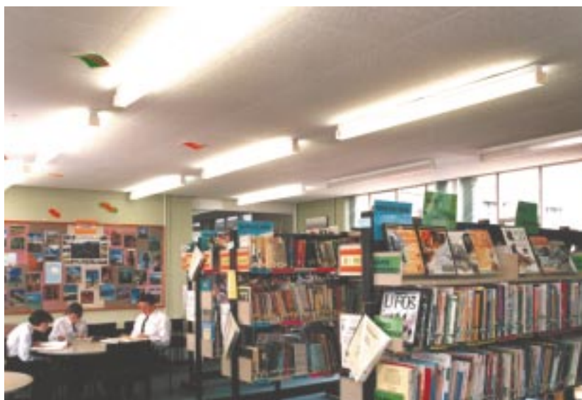
Figure 7 New lighting in the library
